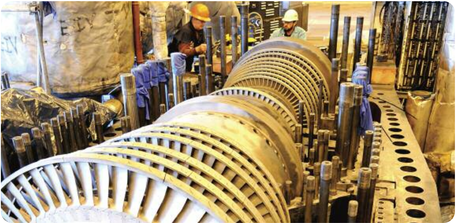
As part of a two-month planned outage at SEC Unit 2, more than 150,000 work hours were invested in maintaining and maximizing the unit's energy output.
