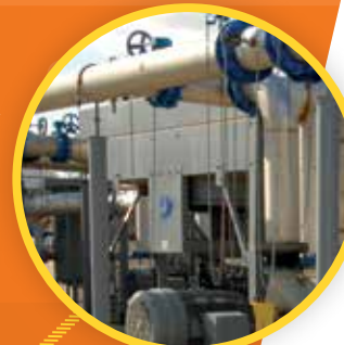
ORANGE COUNTY & HOLOPAW LANDFILL GAS 47 MW
