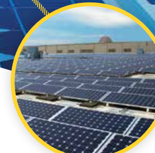
COMMERCIAL ROOFTOP SOLAR
